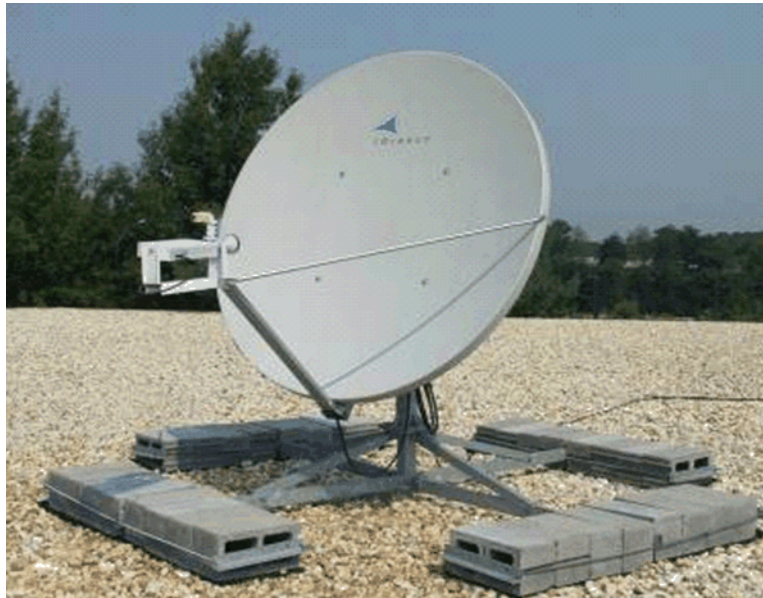
Figure 3. Typical Antenna with BUC and LNB
