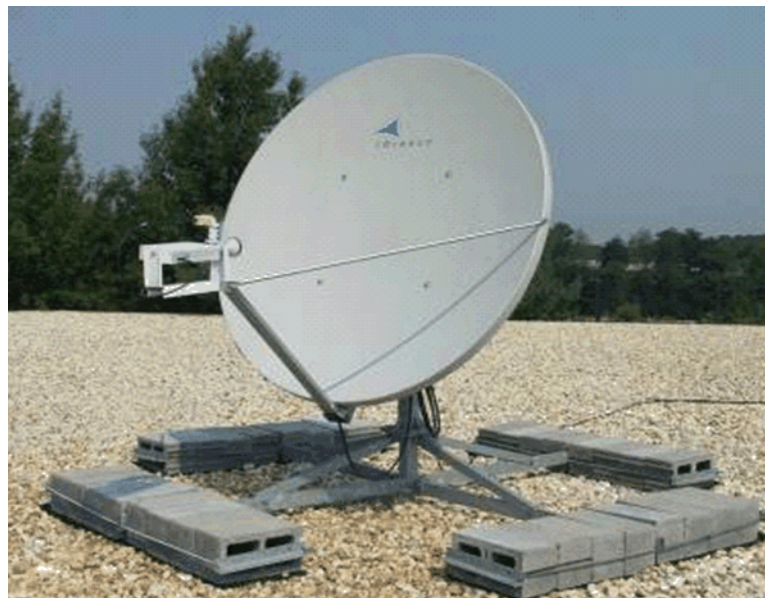
Figure 4 Typical Antenna with BUC and LNB
