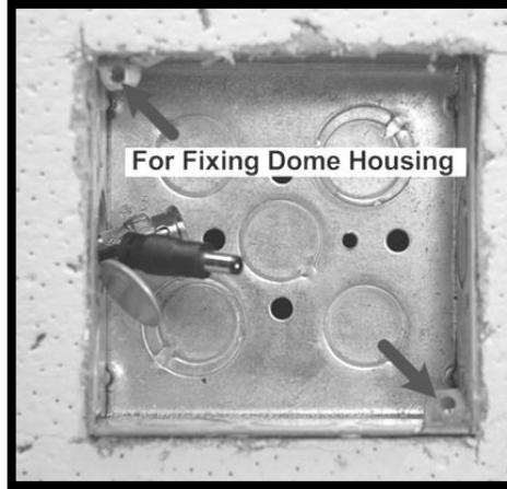
Figure: 4S Mount Electrical Box
