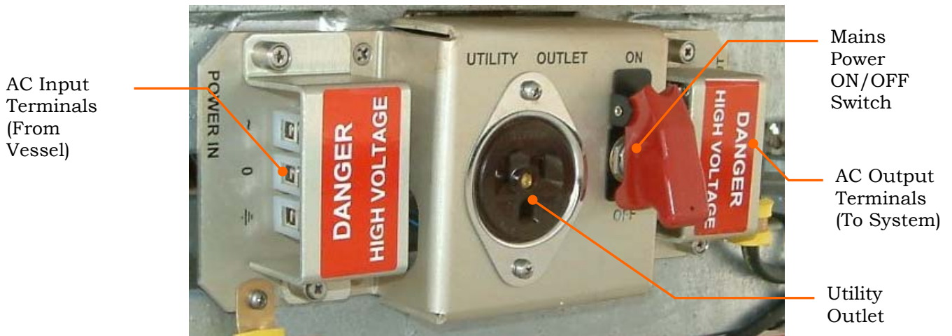
Figure 2-25: ADE Power Connection Box – Original Configuration
