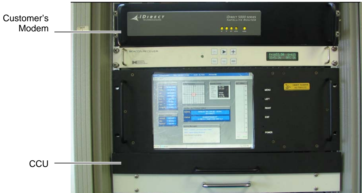
Figure 6-23: Typical BDE Rack Installation
