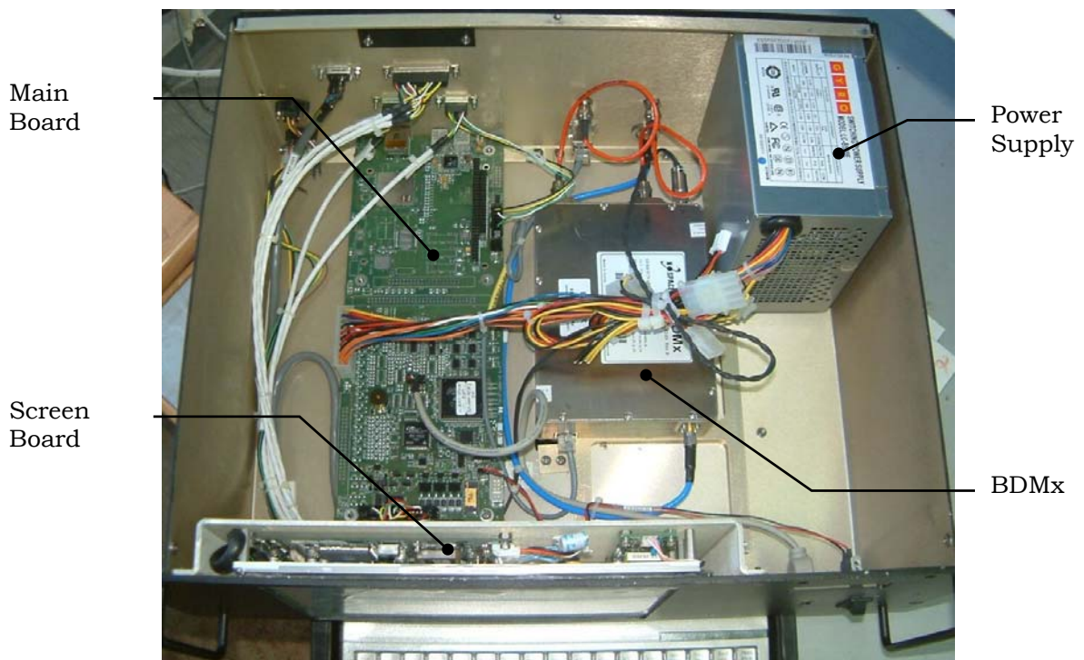
Figure 2-30: CCU Internal View
